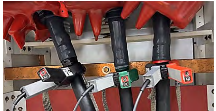
Checking phase consistency from two transmitters before and after operations
